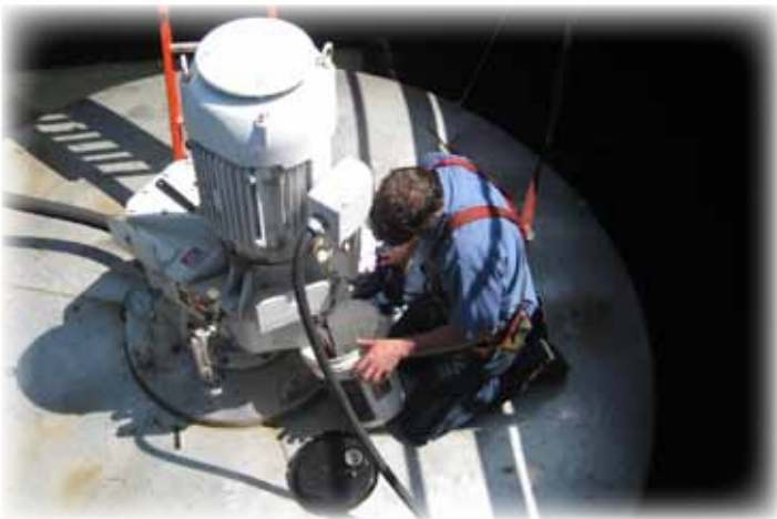
Jamie Piangerelli is seen here draining out the LE gear lubricant that the units were initially filled with.
