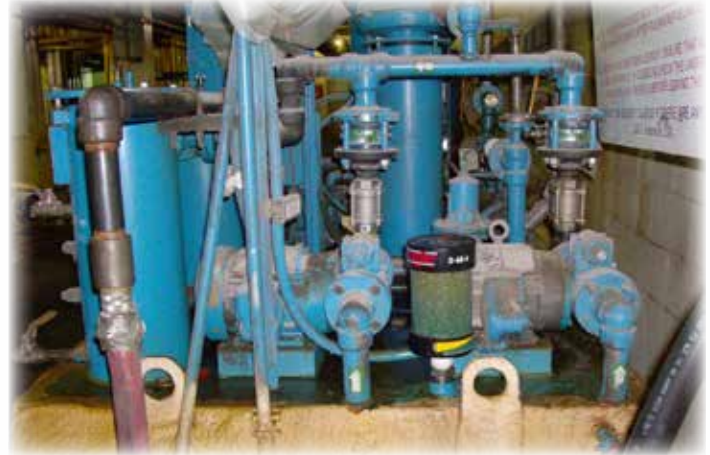
Breather mounted too close to tank
