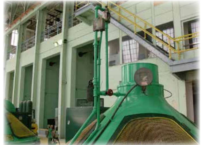
One of six turbines at Ryan Dam
