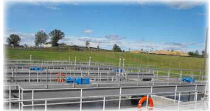
Chemineer mixers in BPR tanks
