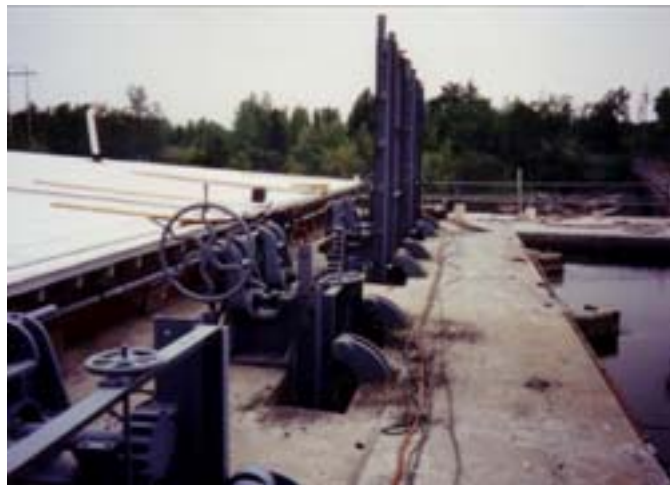
Flow control gates lubricated with LE 4024 QUINPLEX Food Machinery Lubricant
