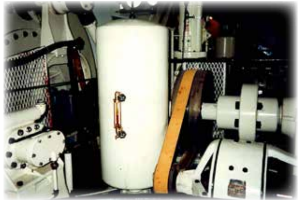
Flow control gates lubricated with Quinplex 4024
