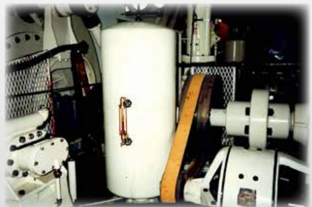
Reservoir for Monolec 6403 to main turbine bearings
