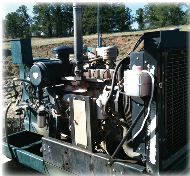
Cummins natural gas engine powered by coal bed methane
