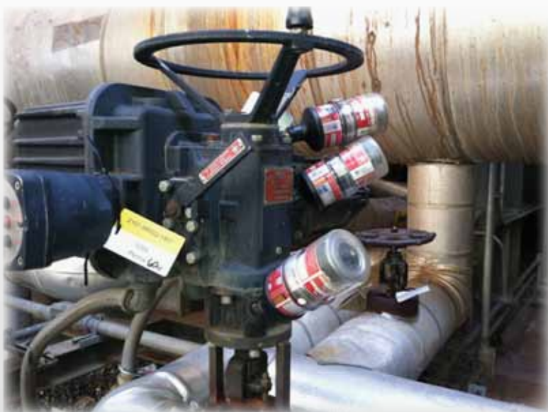
An MOV is shown with multiple grease points using Perma Star Vario 60cc units filled with LE's Almaplex Ultra-Syn Lubricant (1299).
