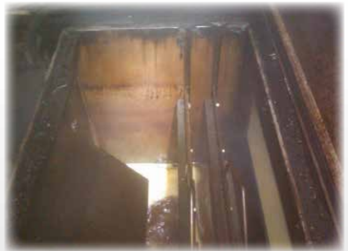
Return line from Bowser oil filtration system
