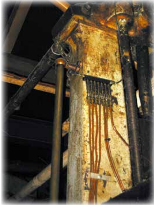
Lube System Manifold
