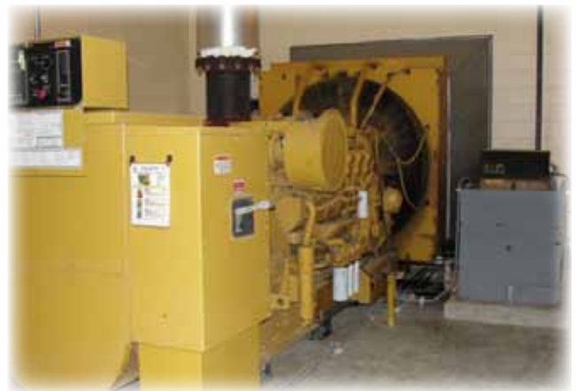
Generator with Cat 3512 engine
