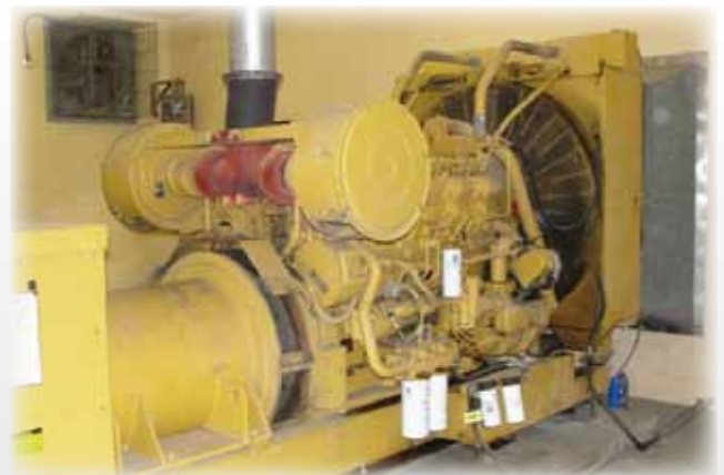
Generator with Cat 3508 engine
