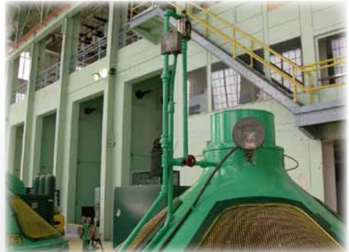
1 of 6 turbines at Ryan Dam
