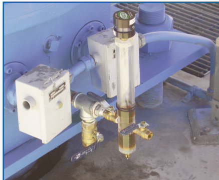
The Esco oil Sight Glass & Level Monitor installed on a gearbox.
